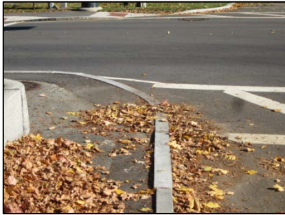
Photo 32: No Curb Ramp at Intersection of Academy Street and North Road.
