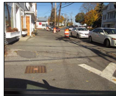
Photo 33: Poor sidewalk conditions in Chelmsford Center. Trees recently removed.
