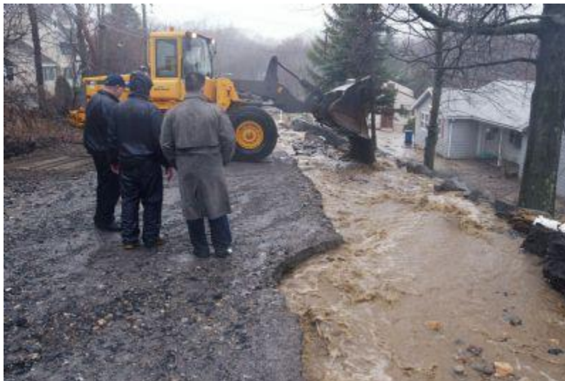
DPW crews work to control roadway undermining created by flooding on River Road in Tewksbury in March 2010
