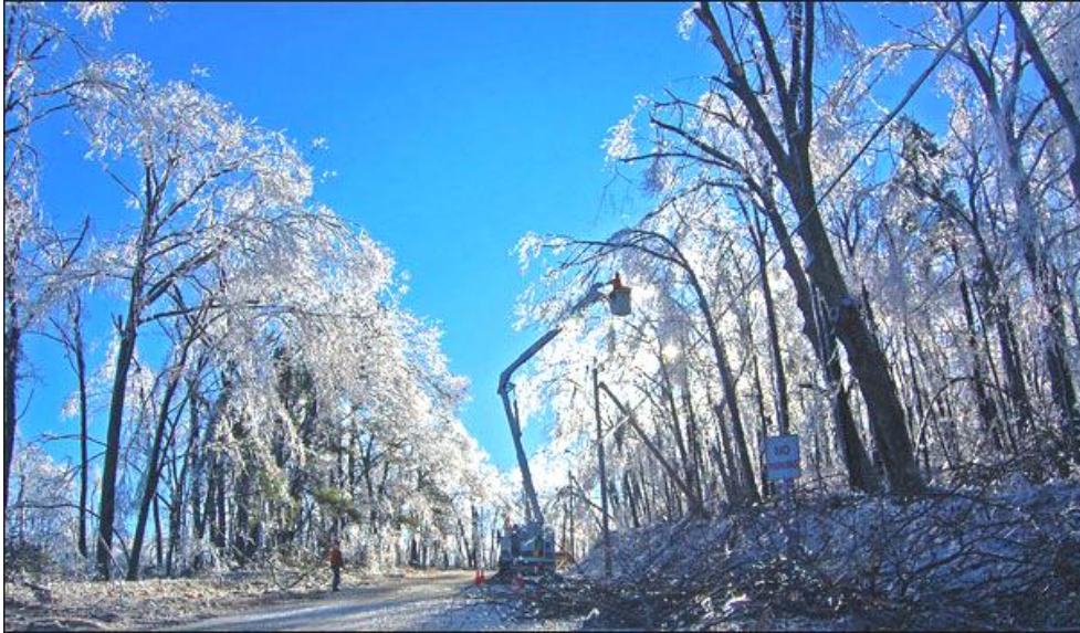
Utility company responds to the aftermath of the December 2008 ice storm in Westford, MA
